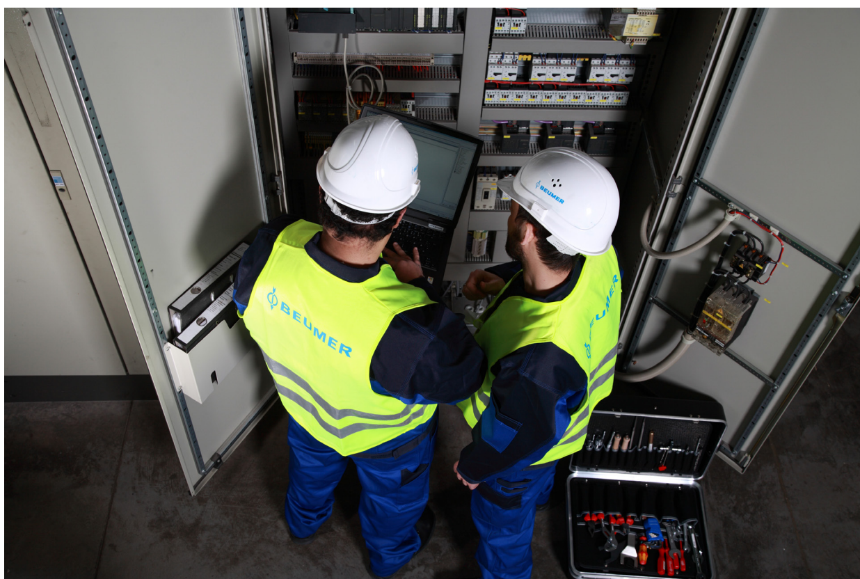
Picture 2: When necessary, the technicians arrive quickly on site to prevent long downtimes.
