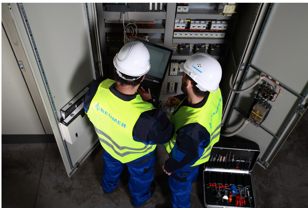
Picture 2: When necessary, the technicians arrive quickly on site to prevent long downtimes.
