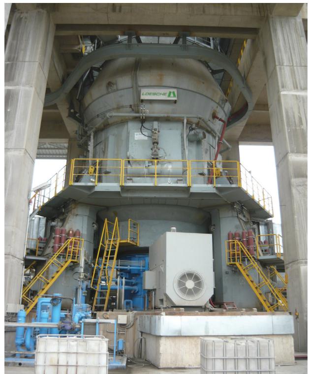
The customer's LOESCHE mill of type LM 53.33+ CS Adana Çimento Sanayii T.A.Ş. at the Iskenderun Cement Works, Turkey.
