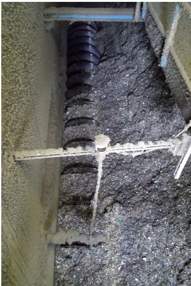
Picture 3: Fill level measuring probes and other measuring technology monitor the automated processes.
