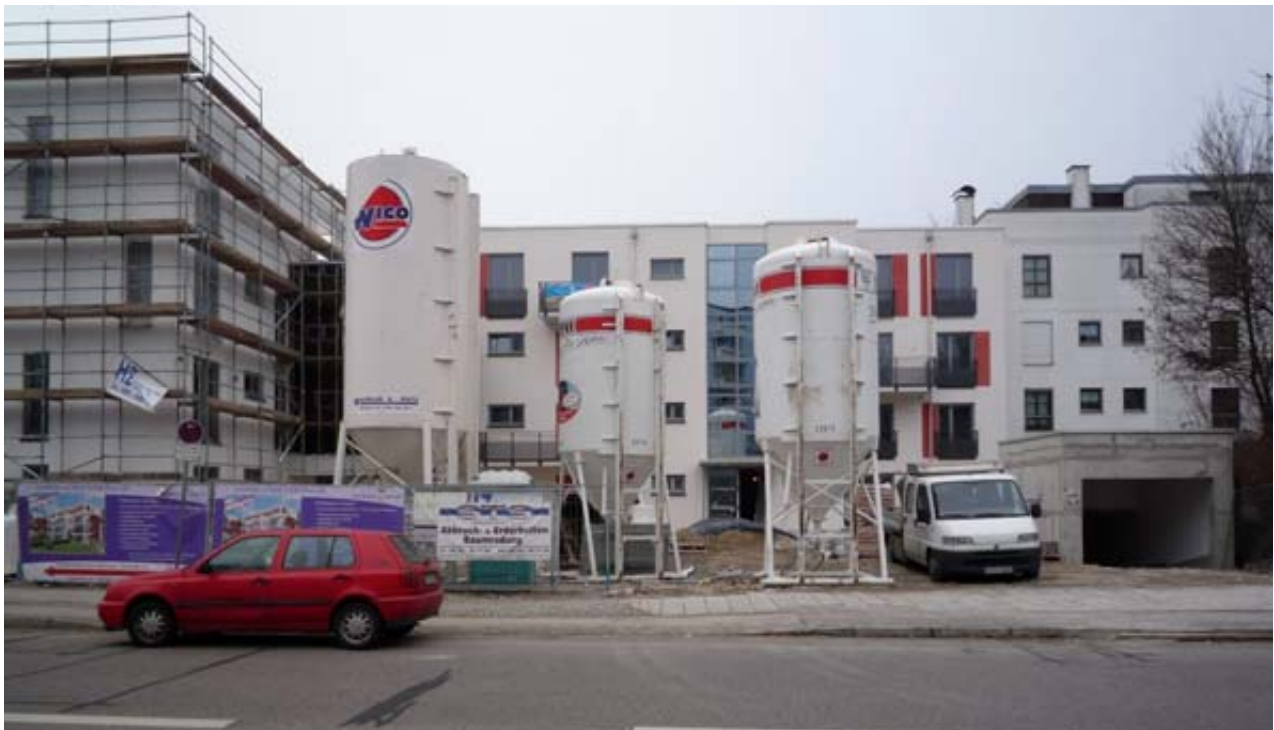
Figure 4: Jobsite in Germany featuring three mortar silos and related equipment. Note the restricted space available in the finishing phase of the construction
