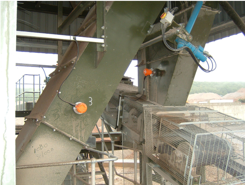
Hycontrol's microwave blocked chute switches in a mining application
