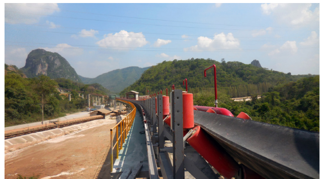
Figure 1: Among other things, BEUMER supplied a troughed belt conveyor with horizontal curves and a length of 3.5 kilometres for the Thai cement producer, the TPI Polene Public Company.
