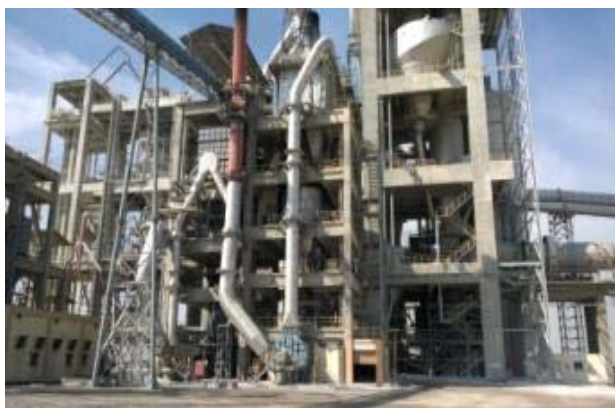
2. In this fuel tower both rotor weighfeeders Pfister® DRW are located and the fuels are dosed and pneumatically sent to the kiln and calciner
