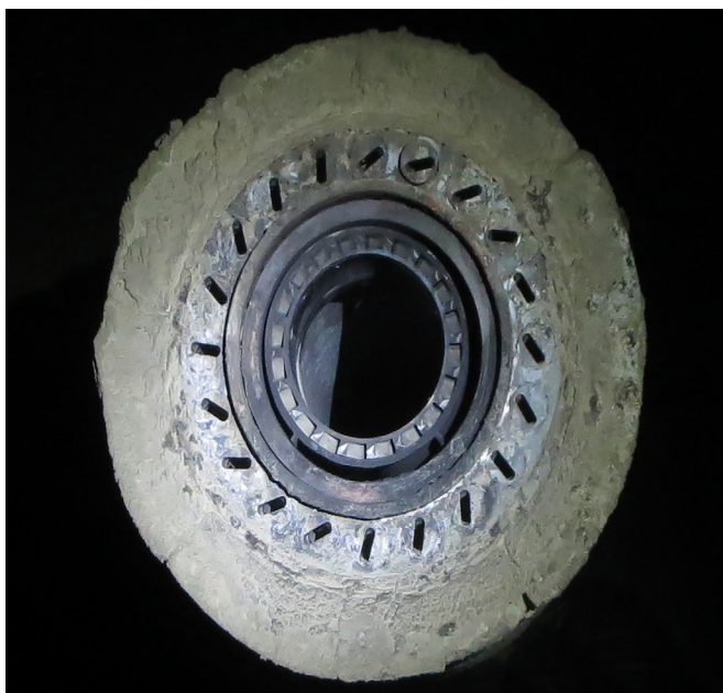
Figure 5: Burner tip in excellent condition after 3 months operation
