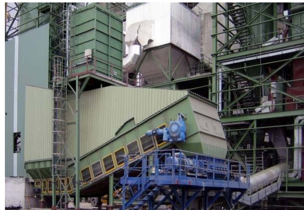
Samson® Gypsum Additions Intake
