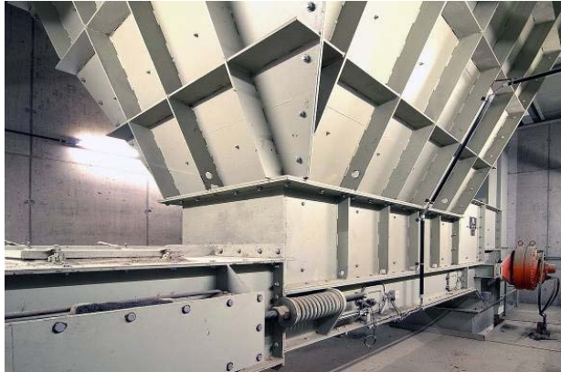
Underground Hopper with AUMUND PKF Feeder
