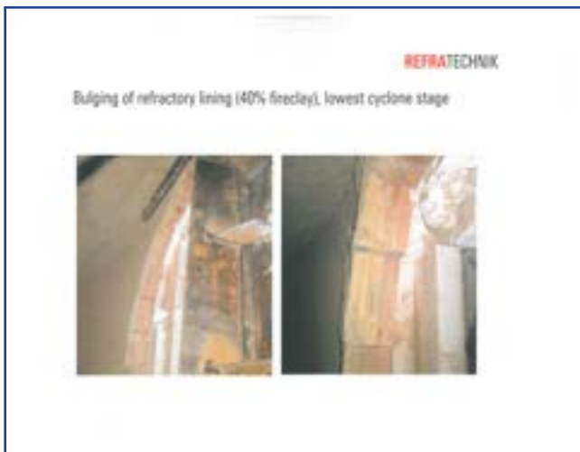
Figure 2: Bulging of refractory lining at cyclone sidewall [2].
