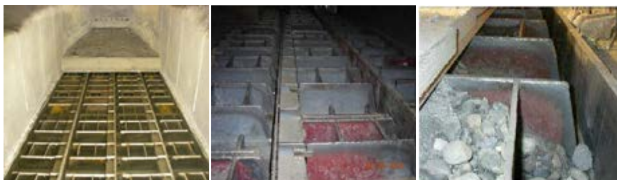
Fig. 4: ETA Cooler Siggenthal at installation/after 4 years/after 7 years
