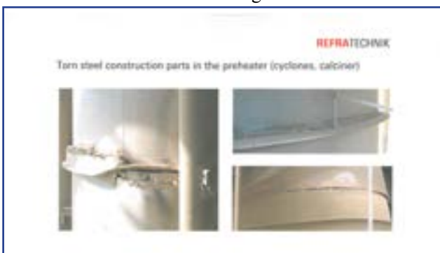
Figure 3: Torn steel construction parts.
