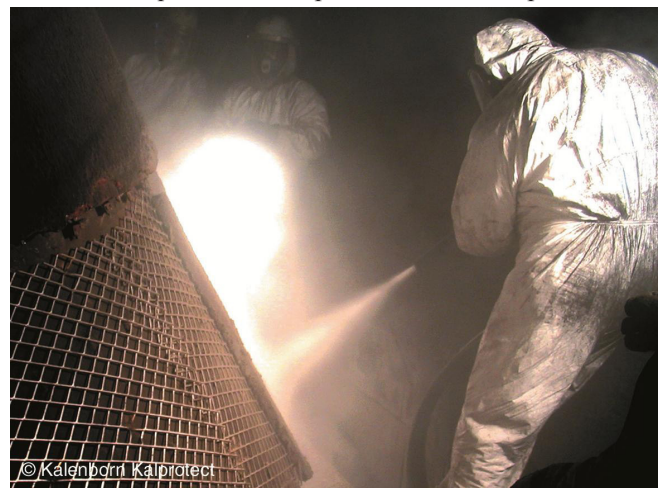
Figure 2 KALCRET-S sprayed on compound enables large surfaces to be covered in minimum of time. The compound can be sprayed on horizontally, vertically and overhead without any problems.
