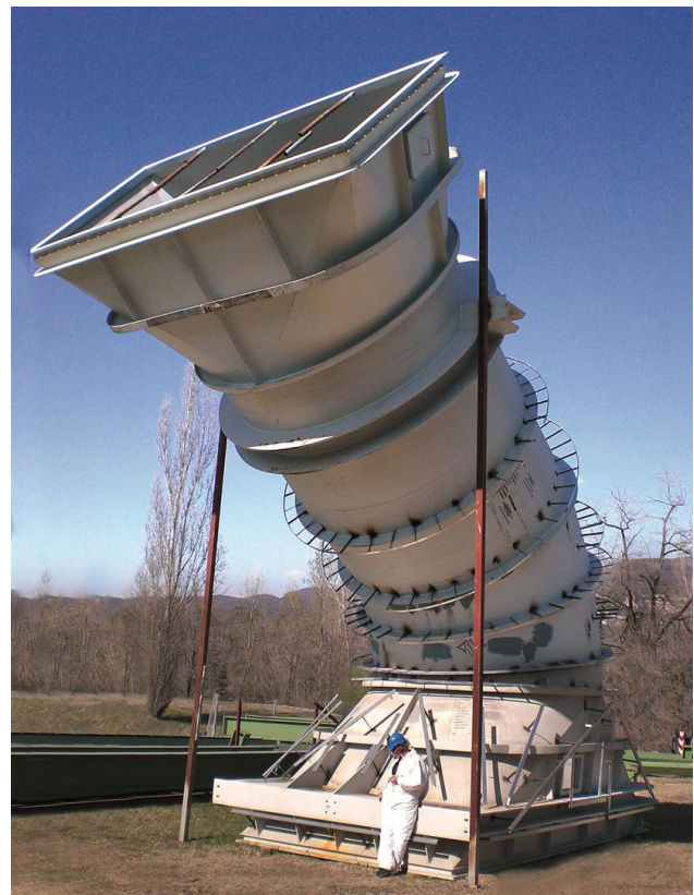
Figure 8 KALCRET-BNX hard compound installed in the discharge bend of the vertical cement mill.
