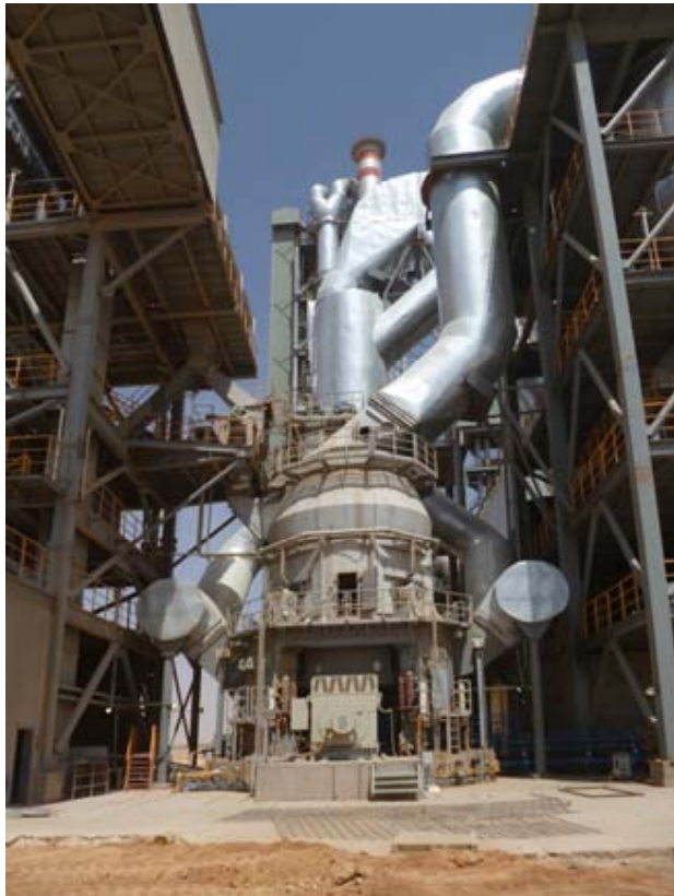
Similar mill type LM 56.4 installed in Hofuf, Saudi Arabia
