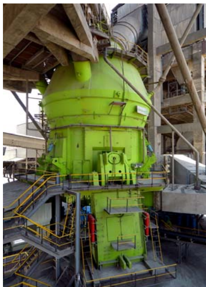
Similar mill type LM 63.3+ 3 installed in Nallalingayapalli, India
