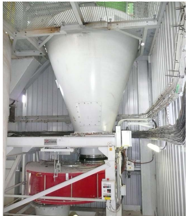
Figure 3A) Installation of a rotor weighfeeder Pfister® TRW-S in the calciner tower
