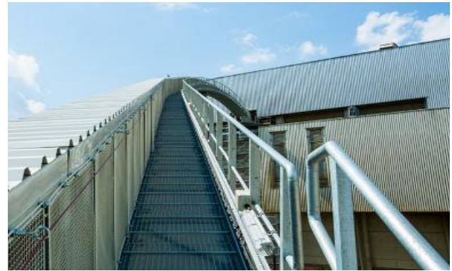
Picture 6: The discharge station shown is at a height of 26 metres. Here the material is transferred onto the feeding system for the main burner.
