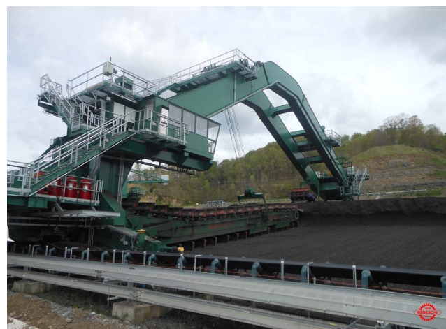
Figure 4: Coal Preblending Storage
