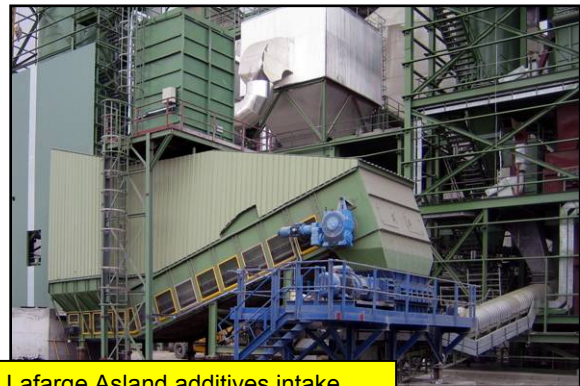
Lafarge Asland additives intake with MMD type 500 rotary crusher
