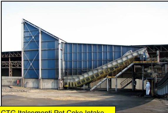
CTG Italcementi Pet Coke Intake
