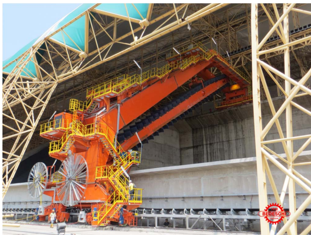
Figure 3: Side Semi-Portal Reclaimer
