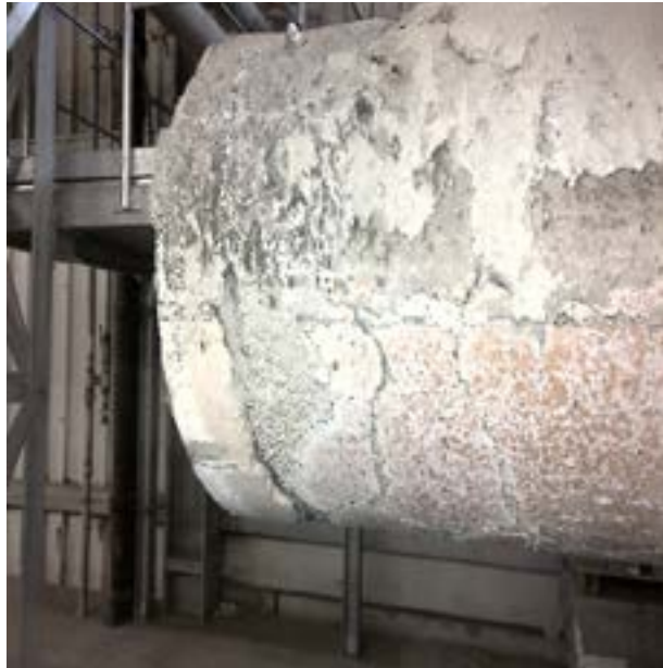
Picture 1: Burner tip lined with CALDE™ MAG BCHC 8004 after 3 months of operation
