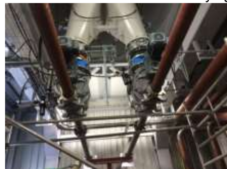
Figure 17: ZXD 300 DP 3 for lignite conveying (Source: Opterra)
