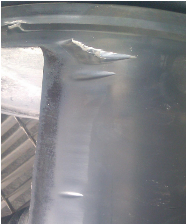
Figure 6: Wear characteristics of flow-control gates
