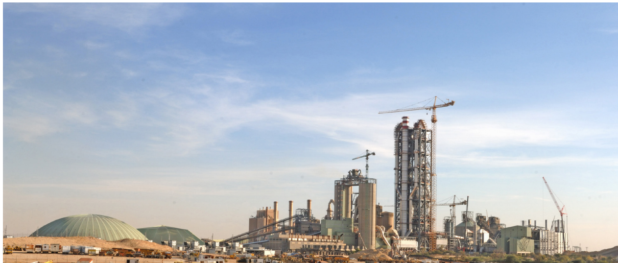
Yamama Cement Company – Existing Plant during Construction Phase of Kiln Line No. 7
