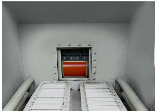
Figure 3: Discharge outlet with flow-control gate
