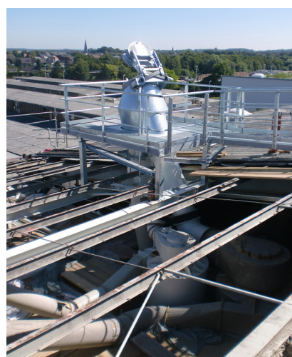
Figure 3: The newly installed explosion vent with explosion pressure relief flap isolates the system and prevents damage to machinery and buildings.
