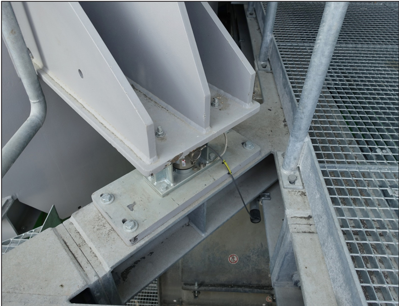
Figure 3- Typical load cell module for silo scales or weighing hoppers
