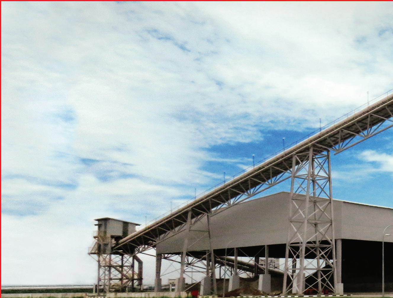
Blast furnace slag silo plant of Meridian Maplestar Sdn. Bhd., Malaysia with IBAU Gdischarge System
