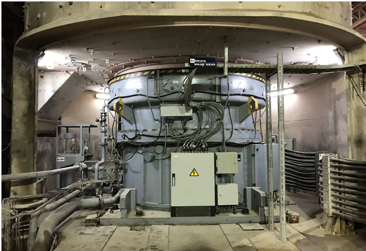
Figure 2: First installation of CEM Drive under a VRM for raw material grinding
