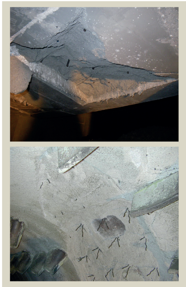
Figure 13: Damage by steam explosions in refractory concrete linings containing cement
