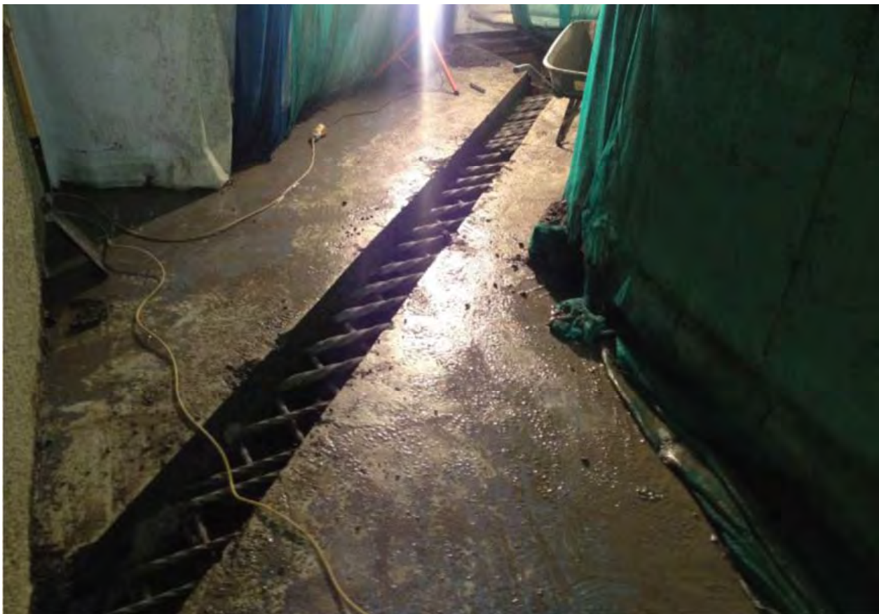
Fig. 2 Rebar's left intact to maintain strength of the floor and surrounding walls
