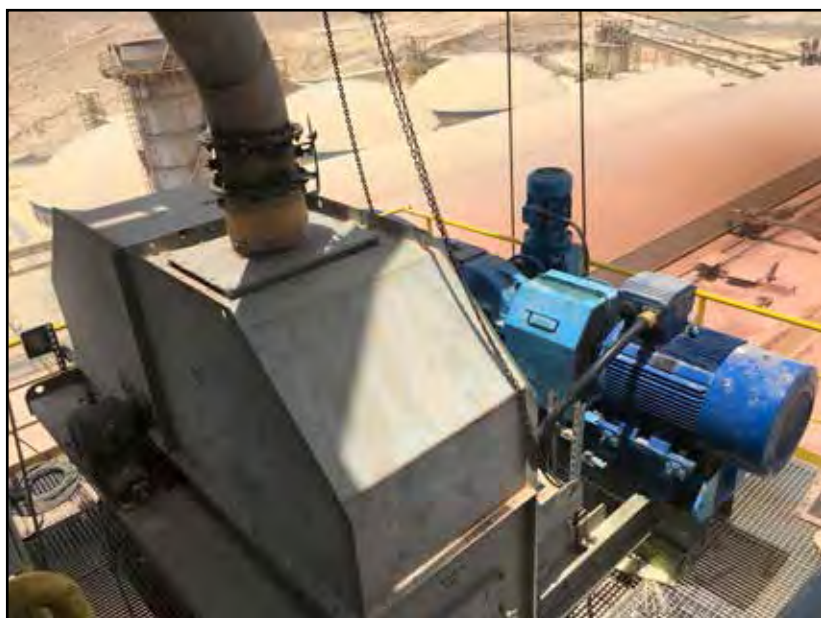
Fig. 3: Desert conditions require everything from the engines of the bucket elevator.
