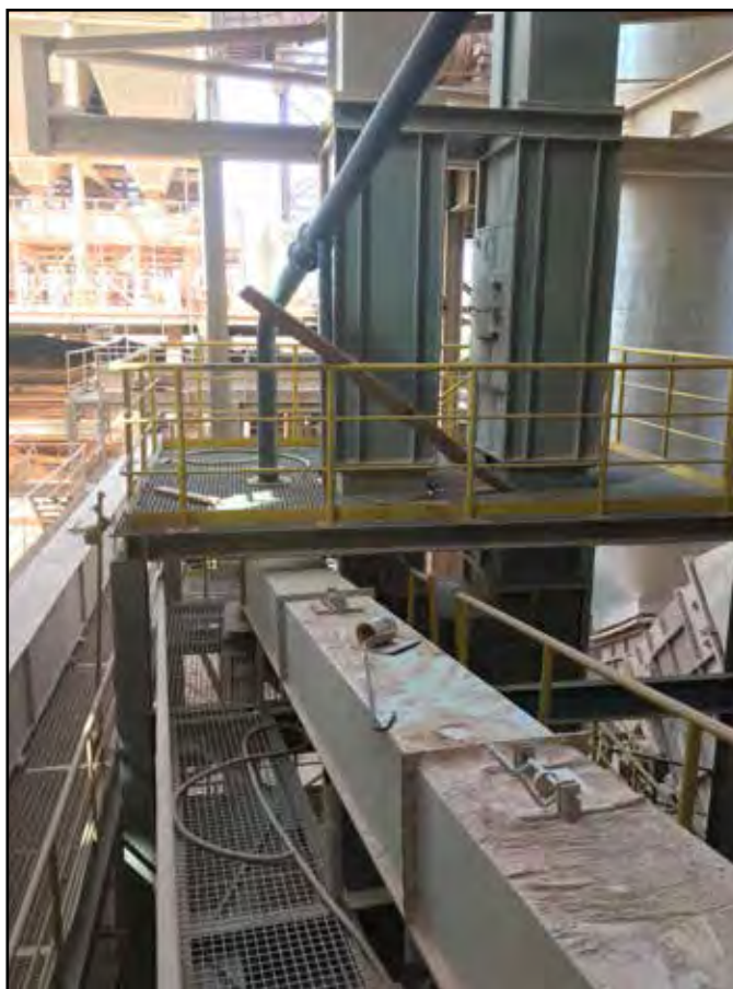
Fig. 2: Installation and commissioning of the new bucket elevator took hardly more than 4 weeks.
