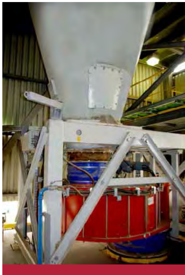
▲ Rotor weighfeeder Pfister TRW-S dosing RDF and biomass to the calciner at Cementos Molins
