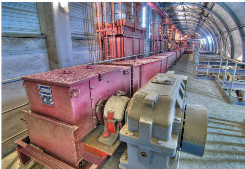
Example application of an AUMUND Drag Chain Conveyor, type LOUISE, in a cement plant (Photo AUMUND)
