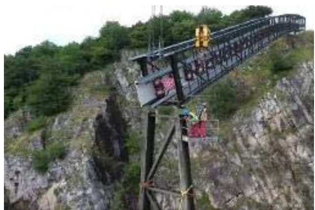
Picture 5: The civil engineering work for conveying systems is usually very complex.
