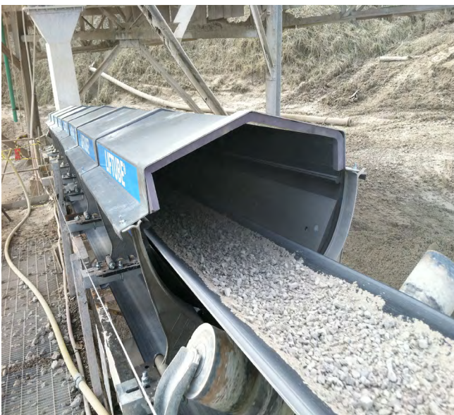
2- Litfube on conveyor
