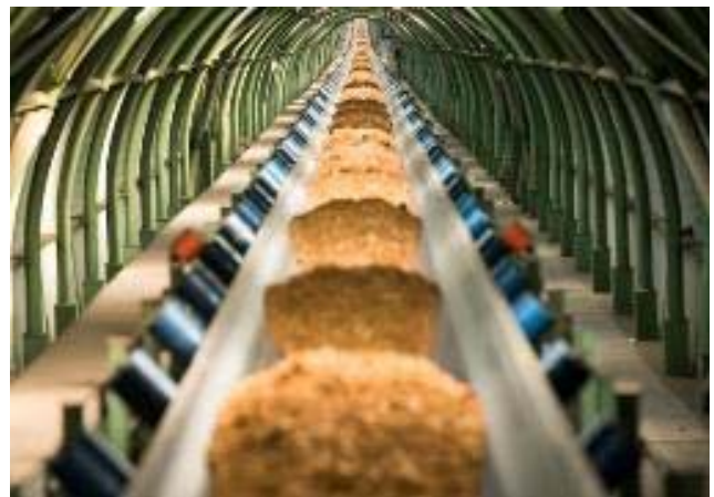
Picture 4: View of the enclosed conveyor flight in the area of the bridge
