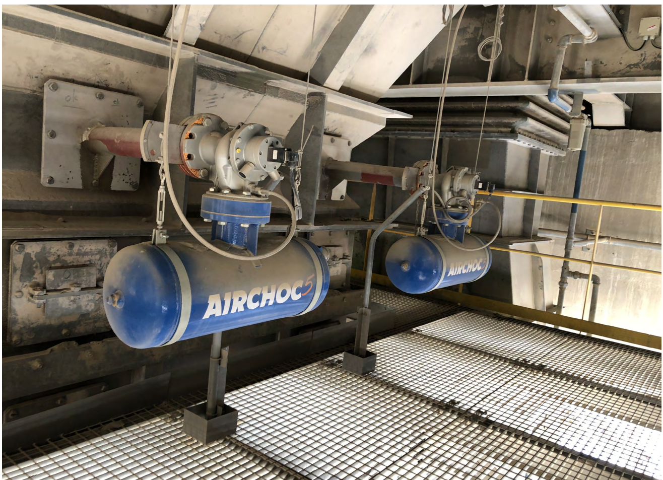
3-Airchoc on cooler
