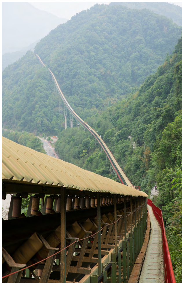
Picture 3: Sichuan project: The troughed belt conveyor runs through rough terrain and over instable ground.
