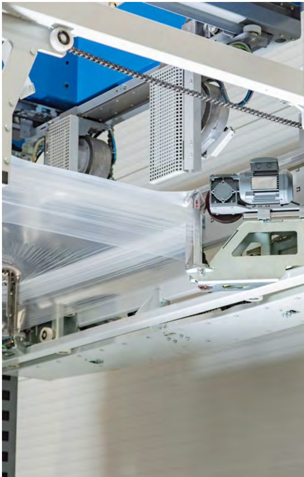
Photo 3: The palletised goods can be forwarded to the packaging system through the roller conveyors.
