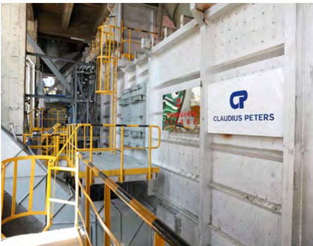
ETA Cooler. Plant: Shanshui Pingyin Line #2, Clinker Capacity: 6500 t/d, in operation since April 2020.
