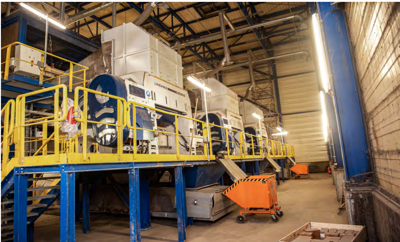
Three Polaris 2200 machines prepare the waste for energy recovery at the power plant. Copyright Lindner Recyclingtech
