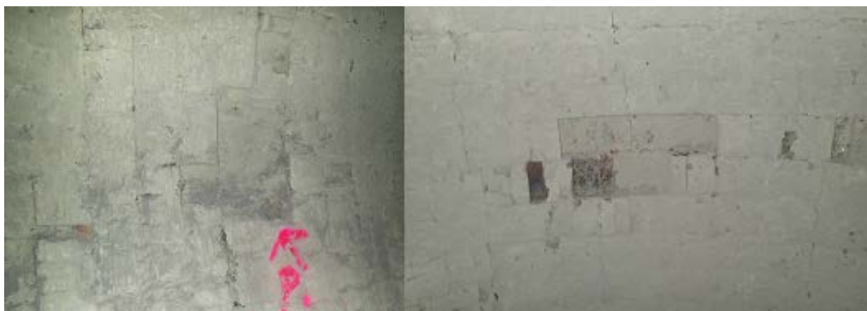
Figure 1: Brick “capping” due to shell ovality (BZ/upper transition – Tyre 2 spinel bricks)
