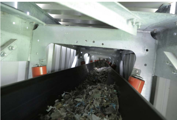
Picture 5: Inside of a U-shape conveyor
