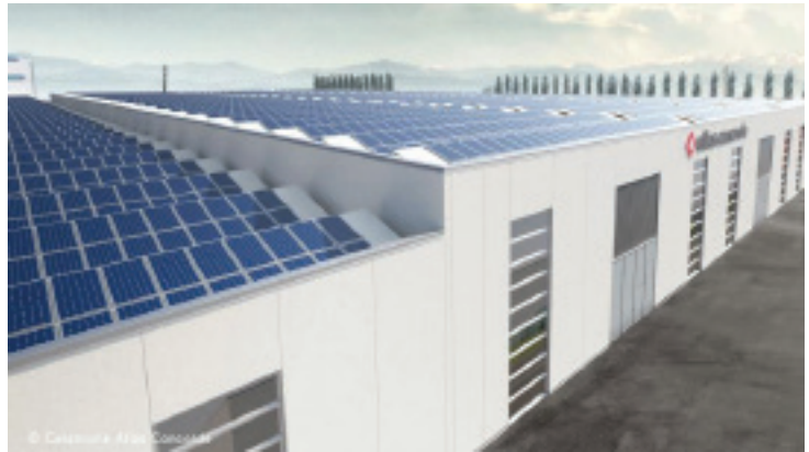
Detail of the photovoltaic system
