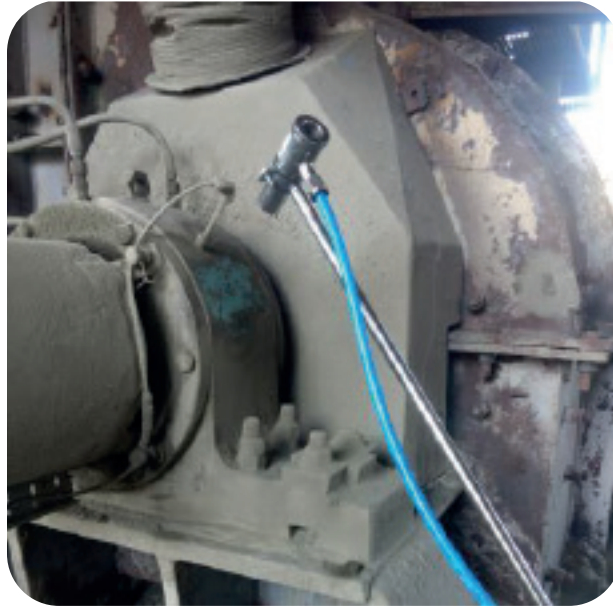
Bearing housing cooling by Energy efficient device (Arrest Master ABS) Input @ 6 Bar = 11 CFM, Output= 77 CFM, Atmospheric contribution= 66 CFM
