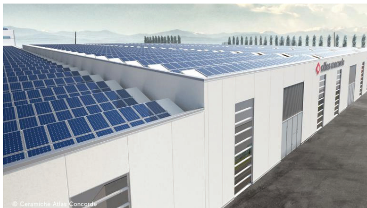
Detail of the photovoltaic system
