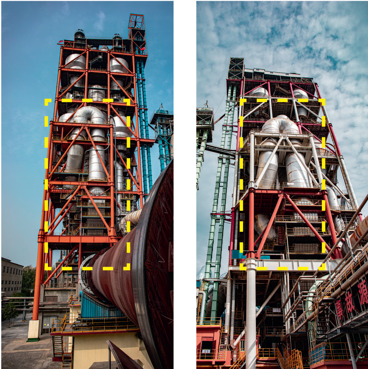
Figure 8: Pyroredox installations in China.
