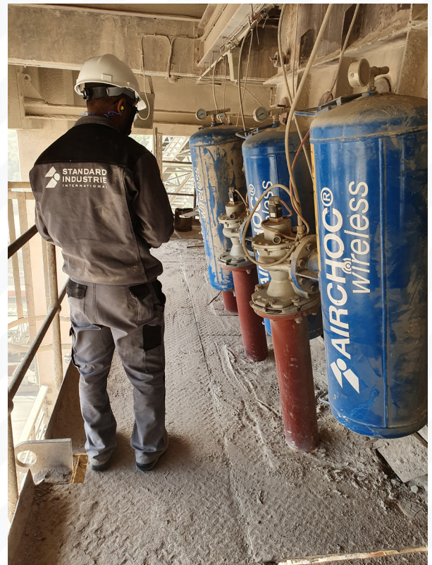
AIRCHOC air cannons on smoke box in cement plant
