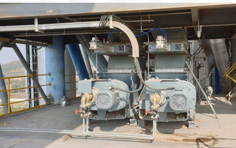
prepol® SC connected to the lower calciner section
