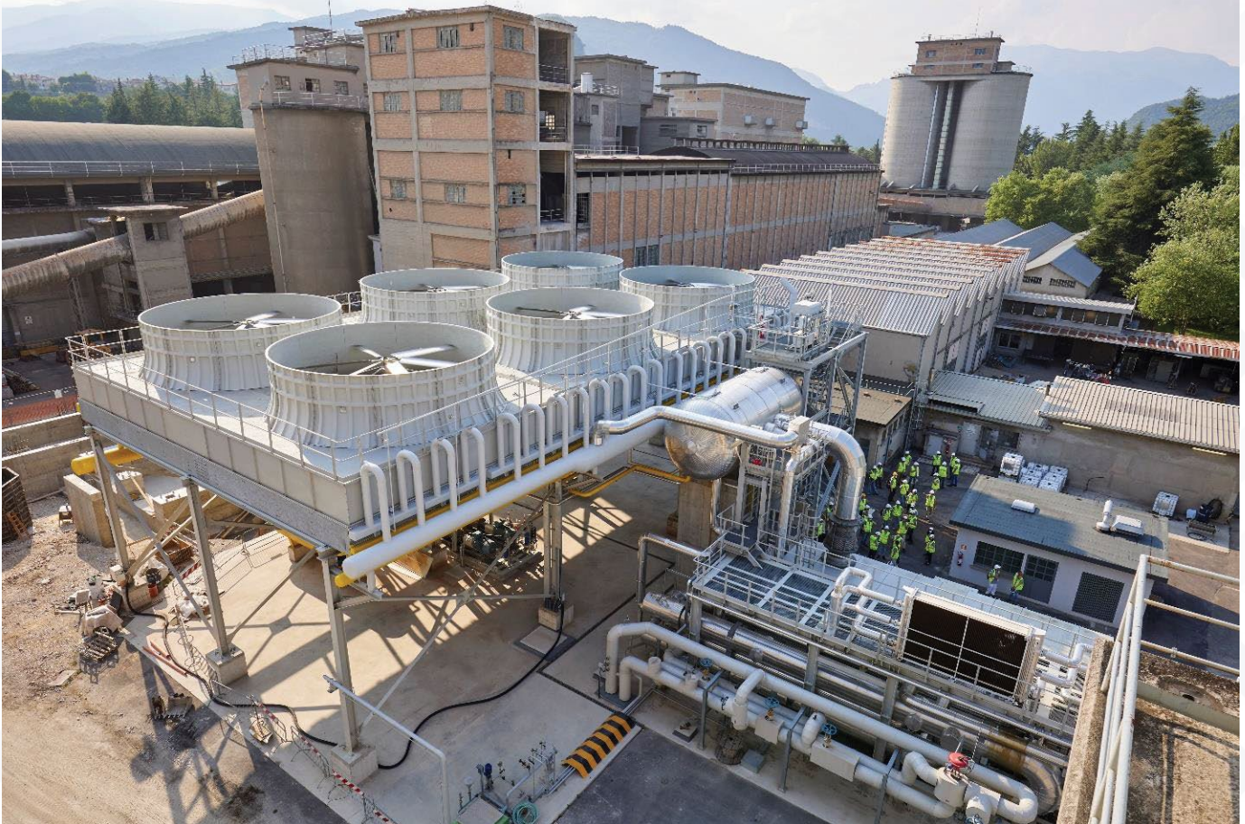
Figure 4. A view of the ORC power plant in CementiRossi cement factory
