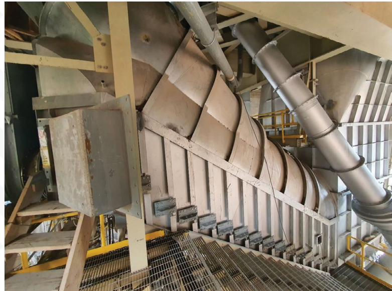
prepol® SC connected to the lower calciner section
